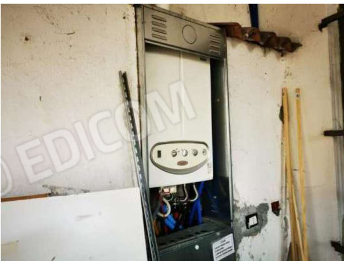
Caldaia a gas
