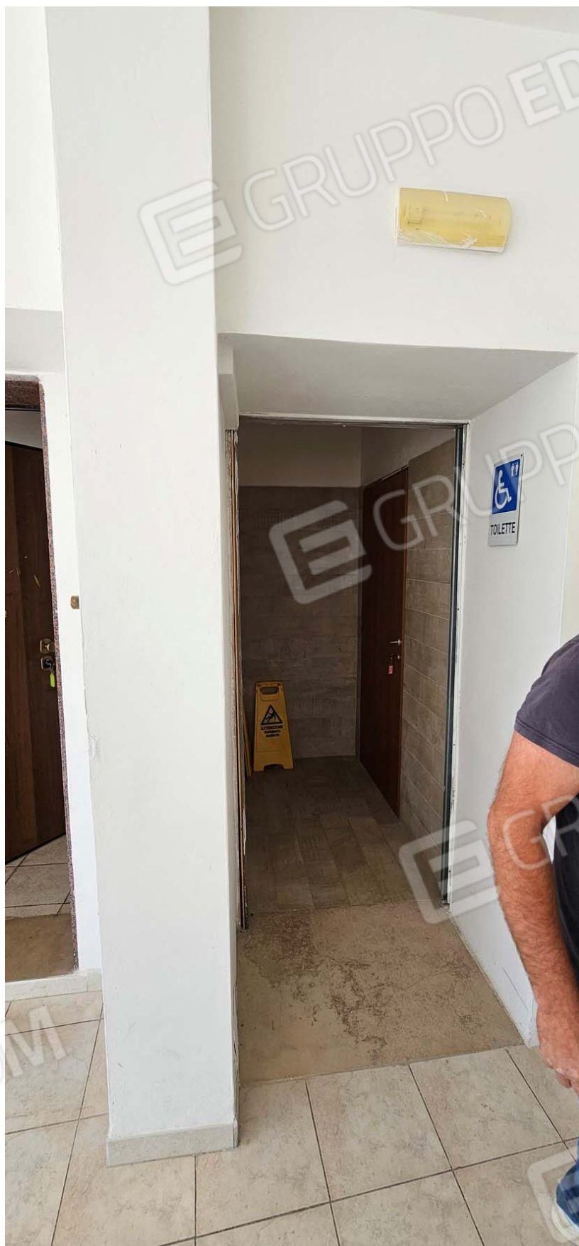
Vano difforme: bagni piano terra
