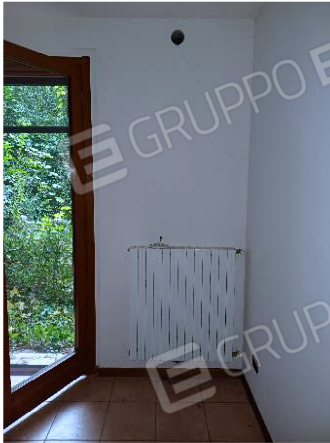
Termosifoni in ghisa
