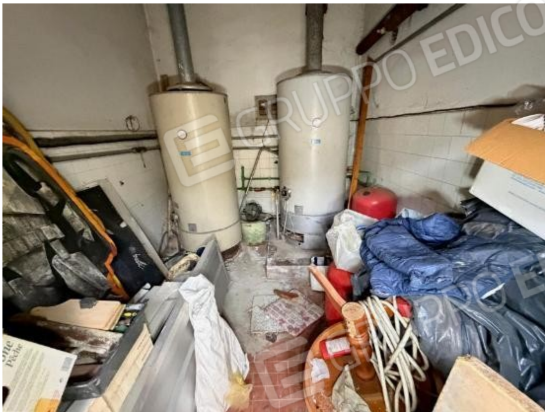
Accumulo ACS in disuso
