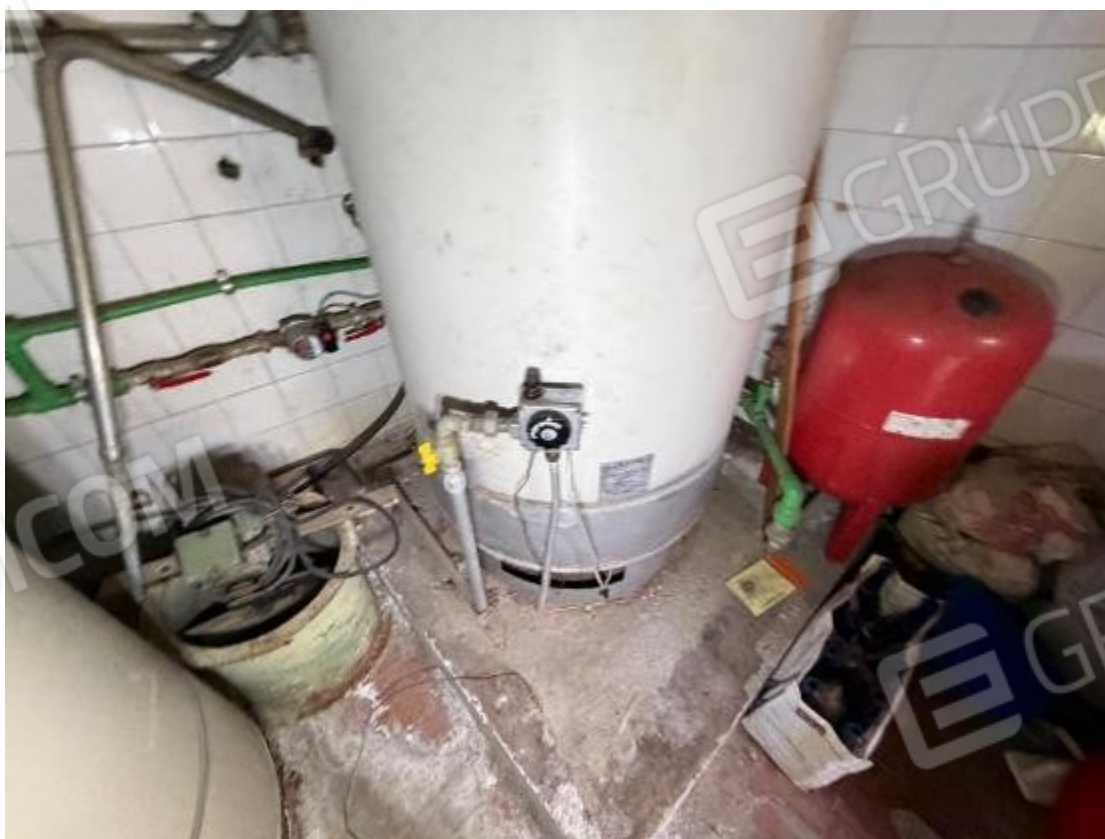
Accumulo ACS in disuso
